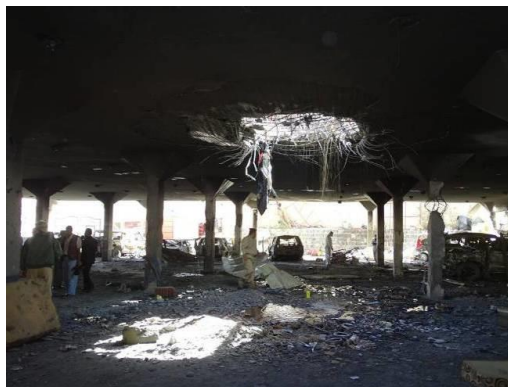
Figure 49.D.3 Post blast interior
