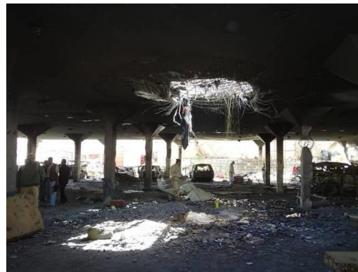
Figure 49.D.3 Post blast interior
