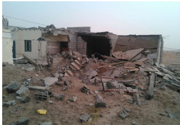
Figure 49.B.3 Armed group suspect's house post-explosion
