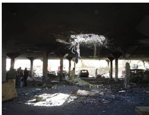
Figure 49.D.3 Post blast interior
